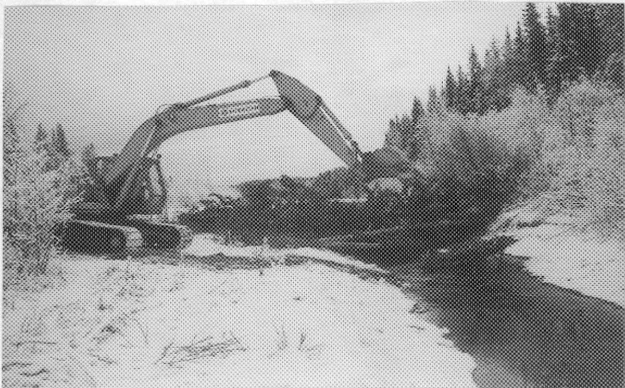
Photo 5: Typical Installation of Side Channel Habitat Complexes (1988) Using Backhoe for Placement of Trees Across Channel
