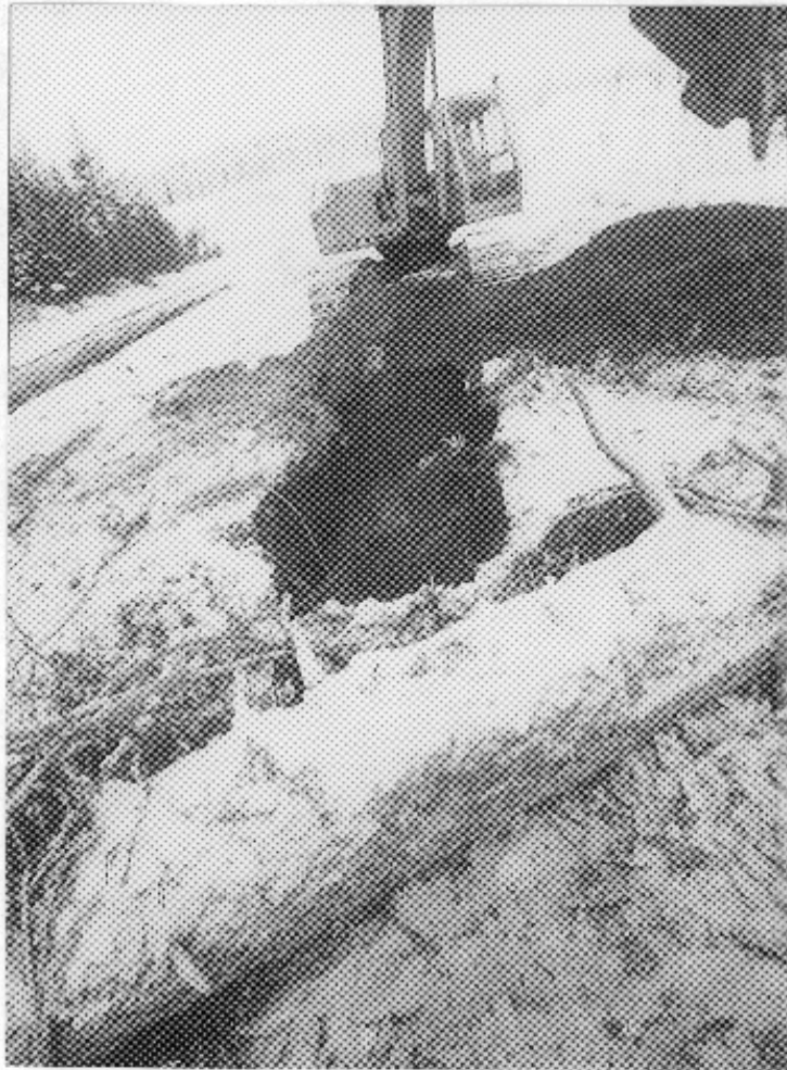
Photo 9: Typical Deadman Anchor Excavation (Cables from habitat complexes were anchored to a 3 m log section which was buried in excavated pit.)
