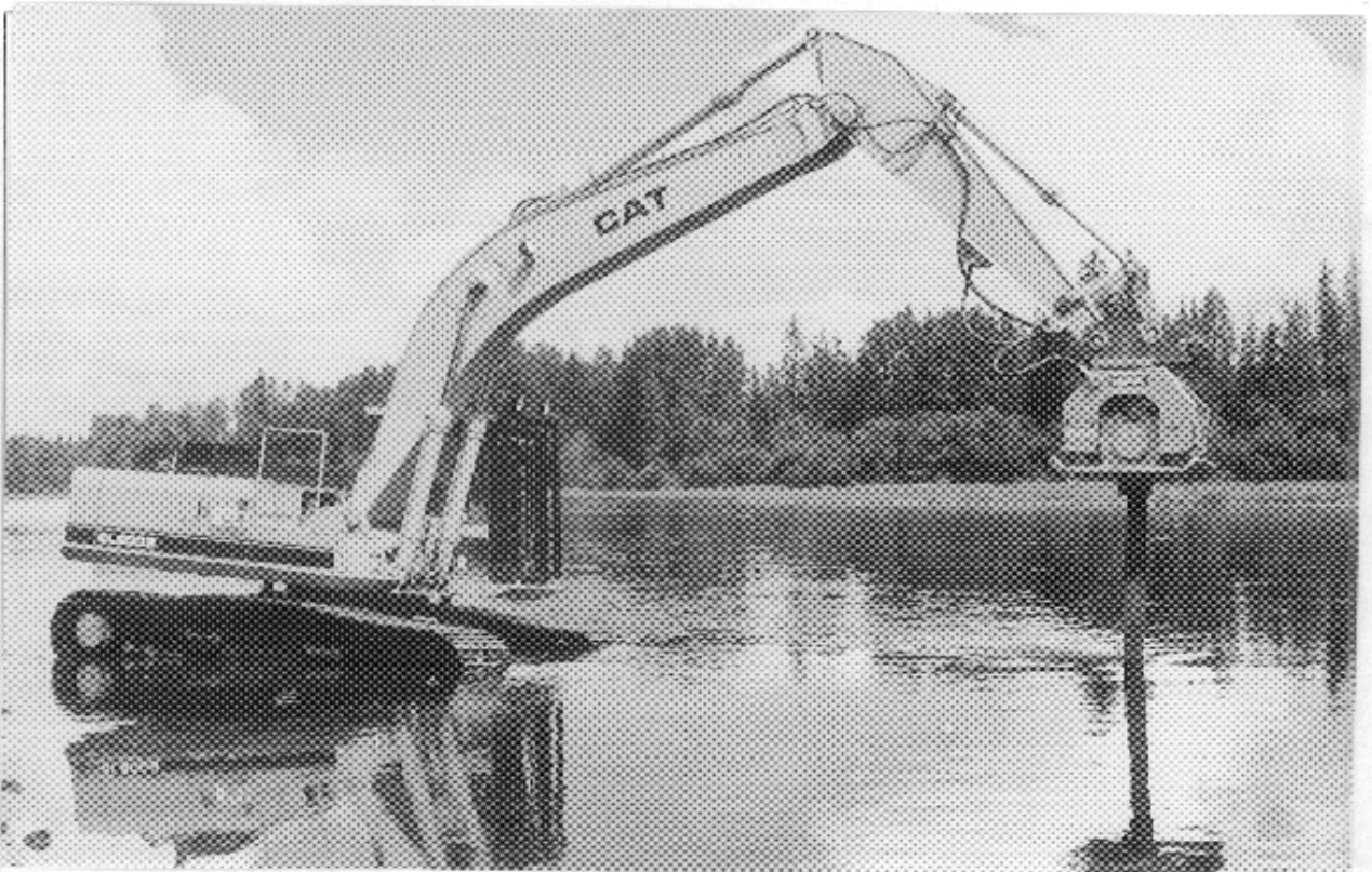
Photo 8: Installation of Rails for Rail Debris Catchers Using a Backhoe Equipped With a Compactor Attachment For Increased Productivity
