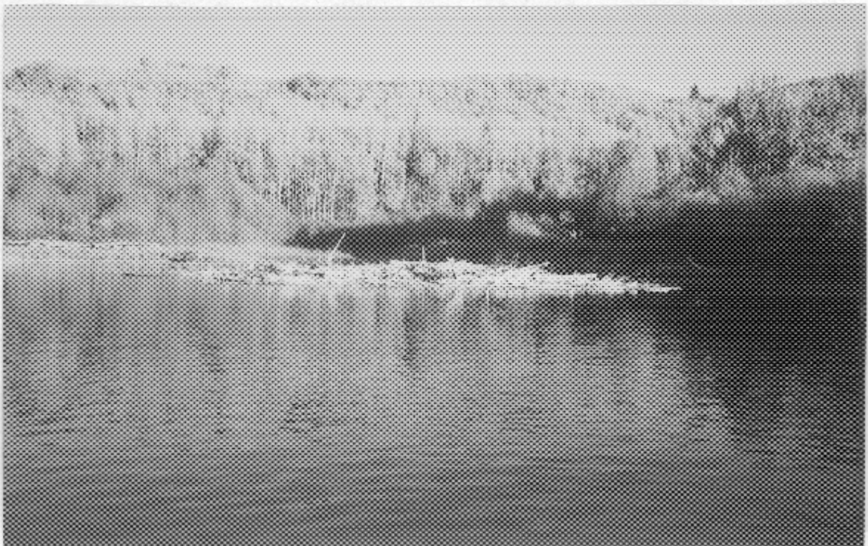
Photo 10: Pipe Pile Debris Catcher (RM35.4PDC) Demonstrating Significant Debris Entrapment
