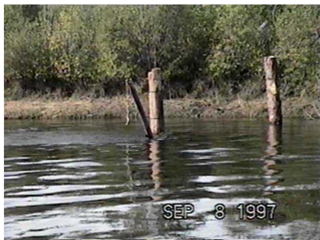
Sept. 8, 1997 – RM86.35 Rail debris Catcher (82.6m 3 /s) Constructed in 1991, this structure captured large amounts of material after construction. The shore debris boom was damaged and much of the captured material was lost. The structure now maintains minimal debris.
