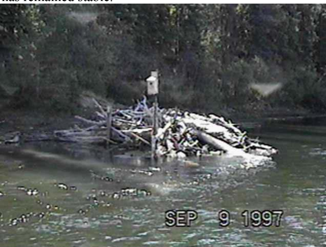
Sept. 9, 1997 - RM 22.55 Rail Debris Catcher (82.6m 3 /s) Constructed in 1991, this structure captured a large amount of material after construction and has remained stable.
