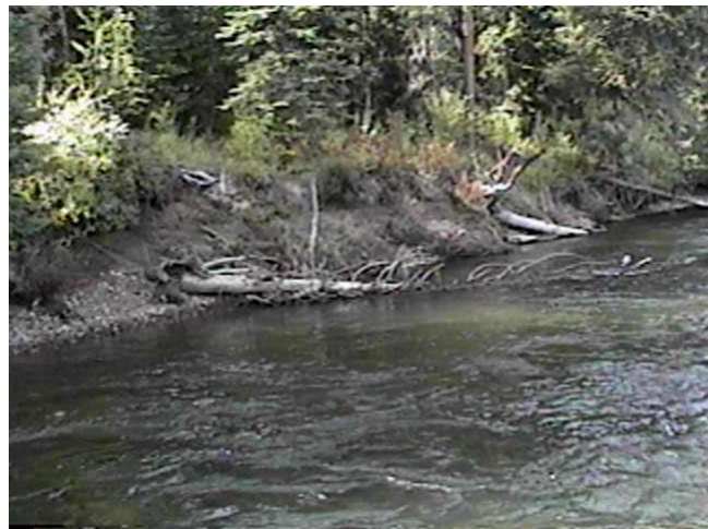
Sept. 8, 1997–LM82.1 Rail Anchored Sweeper (82.6m 3 /s) Constructed in 1991, and modified in 1993 with the addition of a downstream boom, this structure generally fails to trap large woody debris, and has deteriorated over time, and been reduced in size.
