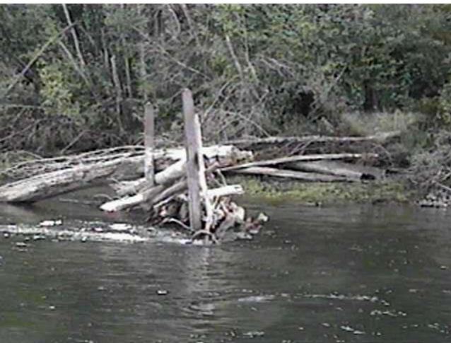
Sept. 9, 1997 - RM16.8 Rail Debris Catcher (82.6m 3 /s) Constructed in 1991, failure of the shore debris boom has also caused this structure to lose most of the debris and prevents the structure from capturing new material.
