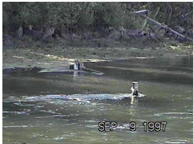
Sept. 9, 1997-RM22.1 Rail Anchored Sweeper (82.6m 3 /s) Constructed in 1991, the sweeper has been broken away from the rails. The rails, which are submerged at high flows are failing to capture woody debris.
