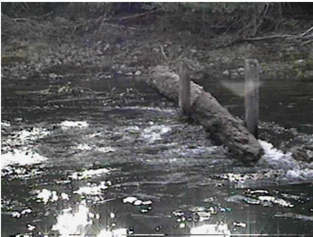
Sept. 9, 1997 - RM16.5 Rail Debris Catcher (82.6m 3 /s) Constructed in 1991, the structures shore debris boom was broken causing the structure to lose most of the debris, and preventing the capture of new material.
