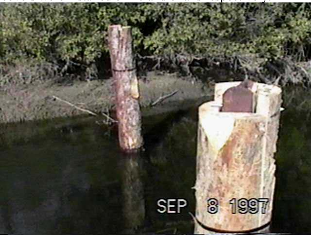
Sept. 8, 1997 – V-Groove Rail Covers To install V-groove rail covers the two halves of the logs were fastened around the rail with banding wire and were bolted through the top of the rail to prevent lifting.
