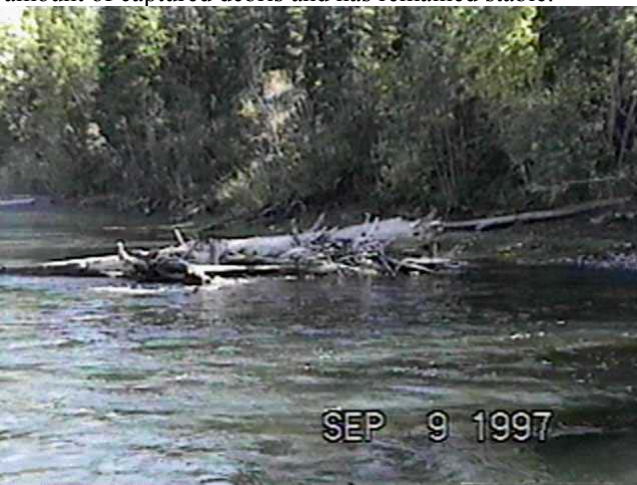
Sept. 9, 1997 - RM22.0 Rail Debris Catcher (82.6m 3 /s) Constructed in 1991, this structure trapped a large amount of debris after construction. Damage to the shore debris boom caused the loss of some material but the structure has remained stable.
