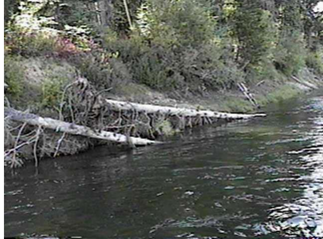
Sept. 8, 1997 – LM82.3 Hand Anchored Sweeper (82.6m 3 /s) Constructed in 1991,, this structure generally fails to trap large woody debris, and has deteriorated over time, and been reduced in size.
