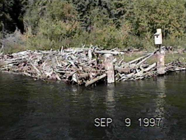
Sept. 9, 1997 - LM21.3 Rail Debris Catcher (82.6m 3 /s) Constructed in 1990 this structure had preliminary debris retention problems, but after three modifications and reseeded efforts the structure has slowly increased the amount of captured debris and has remained stable.
