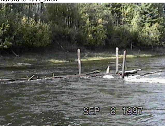
Sept. 8, 1997 – LM 83.0 Rail Debris Catcher (82.6m 3 /s) Constructed in 1991 and modified in 1992 with an additional debris boom from the rails to the shore, this structure generally fails to trap woody debris, and is located in an area of very high velocities.
