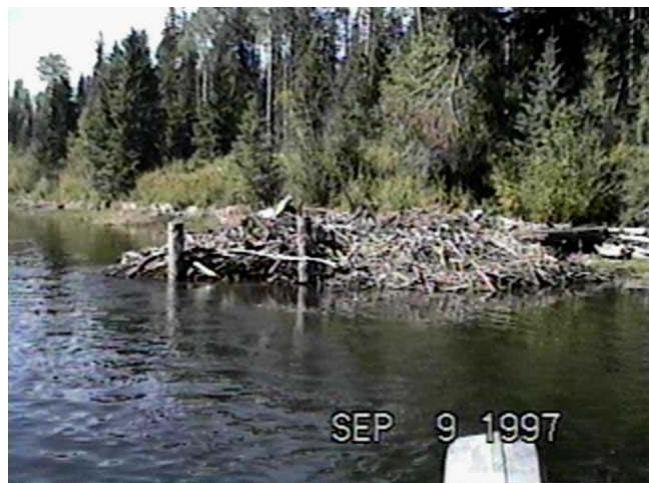
Sept. 9, 1997 - LM22.6 Rail Debris Catcher (82.6m 3 /s) Constructed in 1990, this structure captured a large amount of material after construction and was colonized by beavers. The structure has remained stable.
