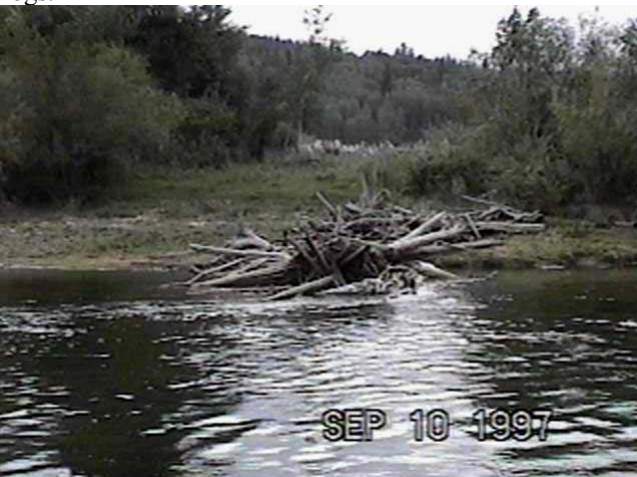
Sept. 10, 1997-RM34.7 Pipe Pile Debris Catcher (82.6m 3 /s) Constructed in 1989, this structure captured a large amount of material after construction, but failure of the outer pipe pile caused a significant reduction in the size of the structure.
