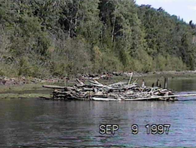
Sept. 9, 1997 - LM 22.85 Rail Debris Catcher (82.6m 3 /s) Constructed in 1990, this structure has slowly accumulated woody debris and continues to remain stable.
